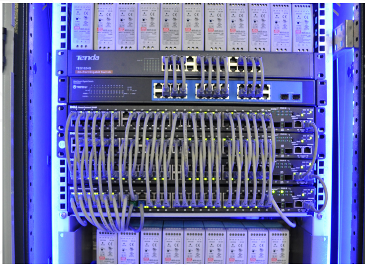
IT Infrastructure Monitoring and Management
